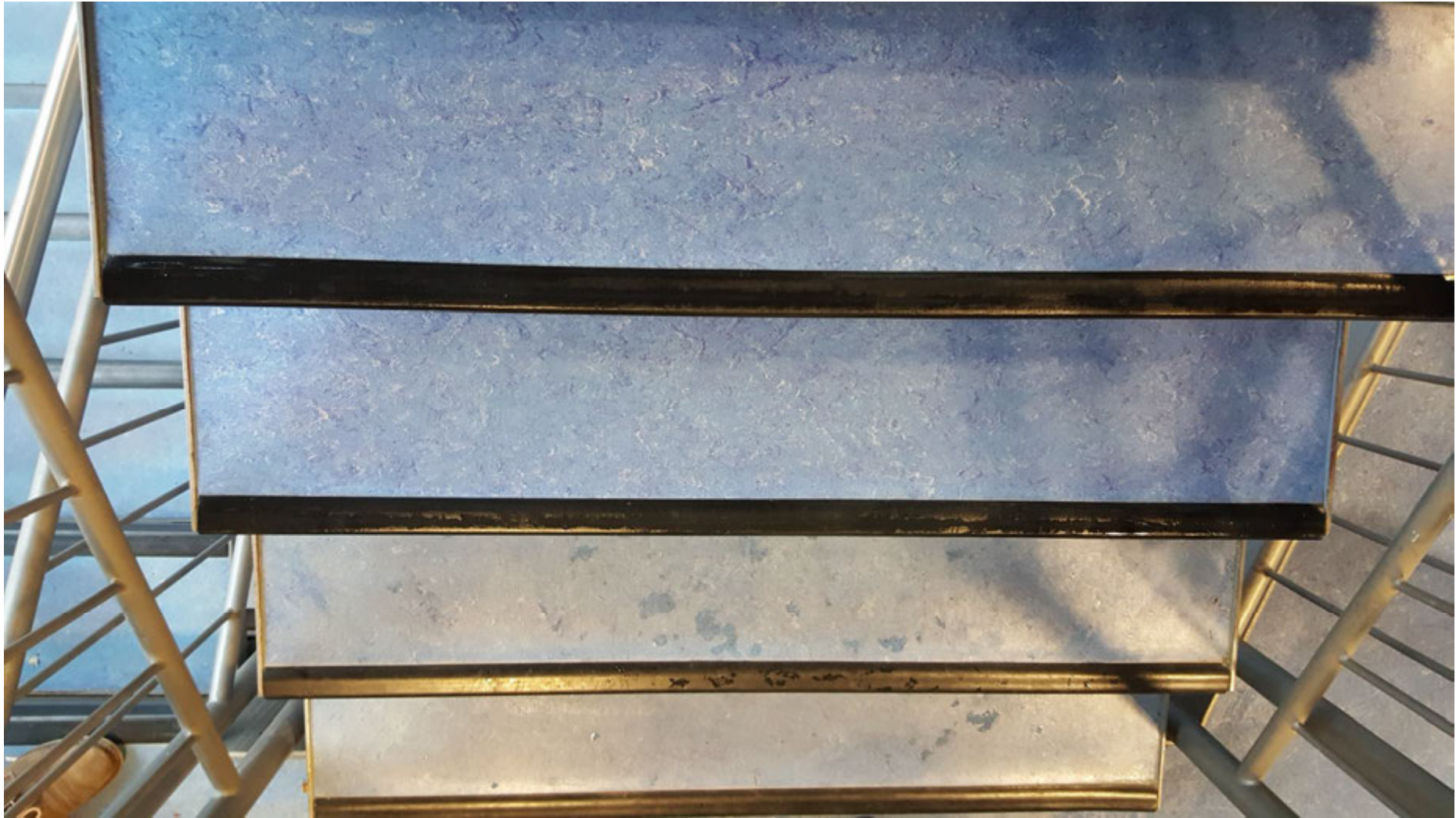
School at Welzheim: Linoleum -Cleaning with Floor Sander Junior and Superfinishing Pad SG 600 (wet)
